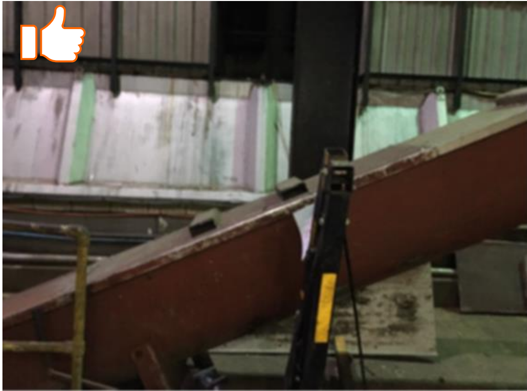
Fully enclosed auger transporting food waste
